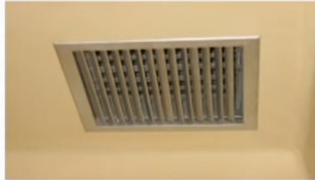
DIFFUSER return grill
