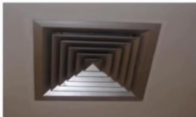
Centralized air condition
